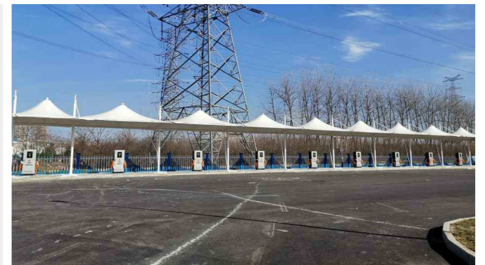
China Tower Project
