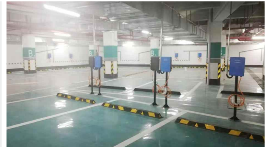
Shenzhen Shajing Charging Station Project
