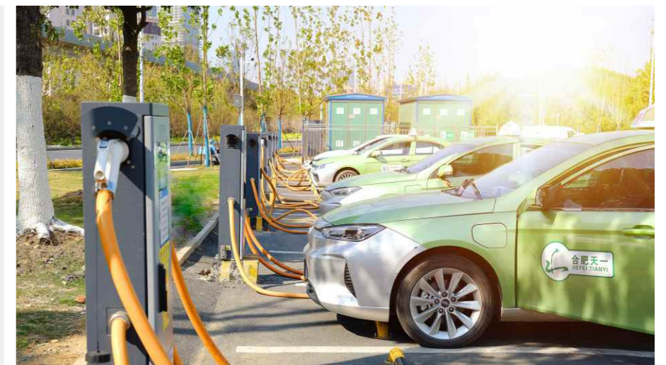
Hefei South Station Charging Station Project
