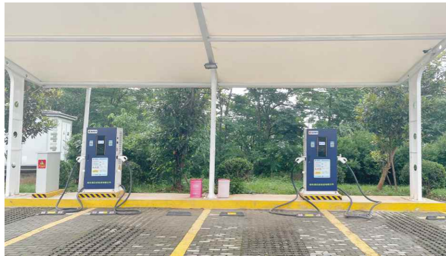
Wuling Power Project
