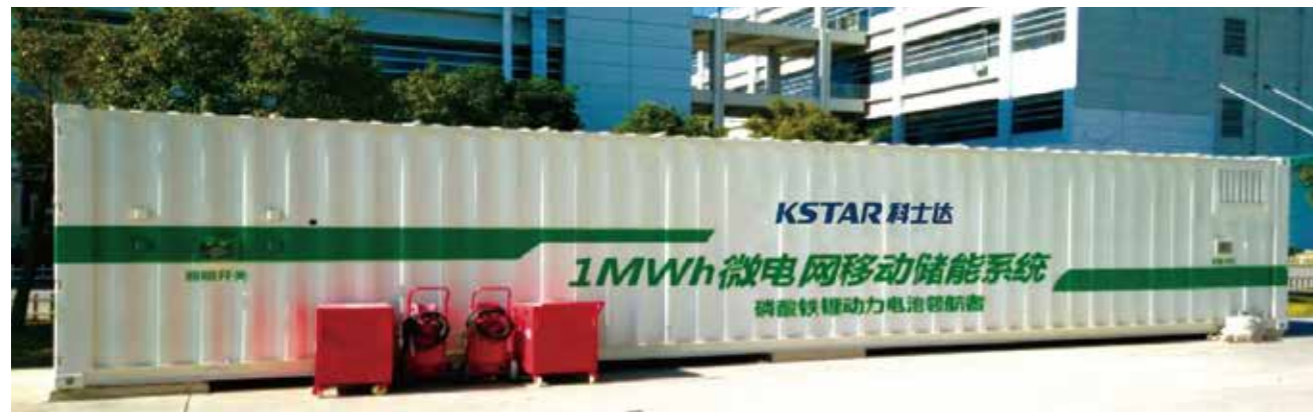
► 3MW/12MWh BESS Demonstration Project in Shenzhen
