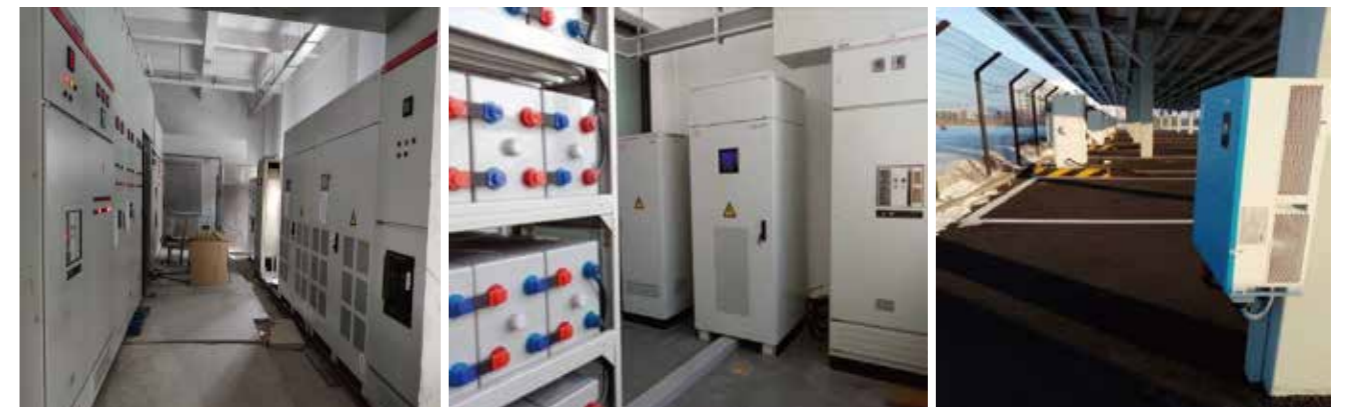
► BESS for EV Charger Station in Harbin
