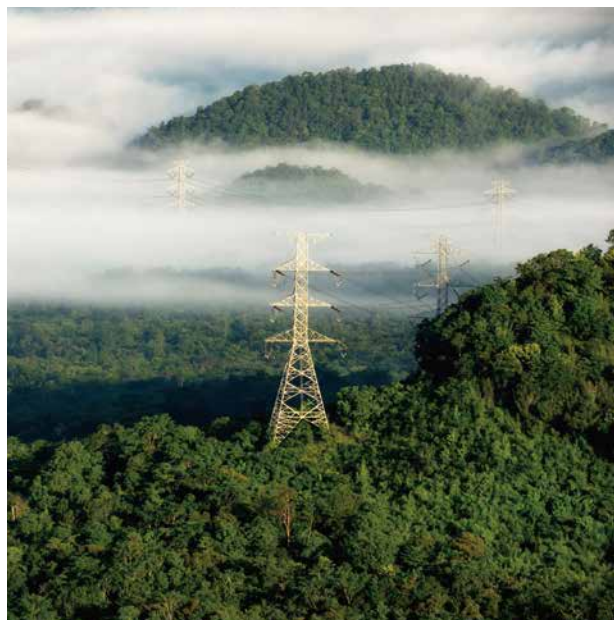
State Grid Project
