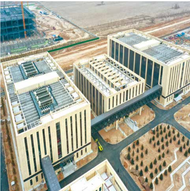
Core Data Center Project for a Major State-owned Bank's Headquarters
