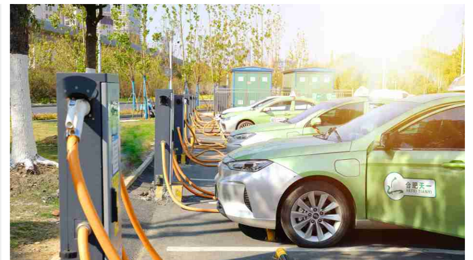
Hefei South Station Charging Station Project
