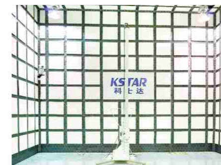
EMI Laboratory (Measuring RE Radiation Interference)
