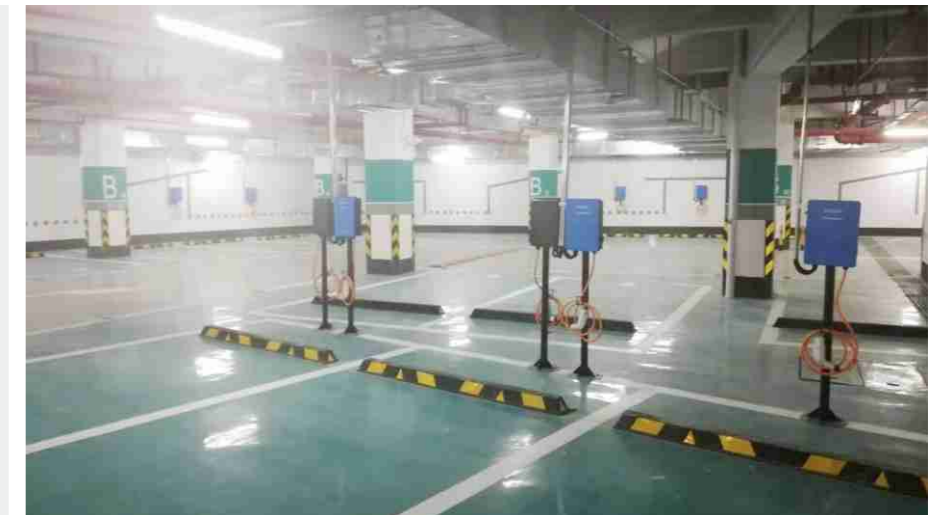
Shenzhen Shajing Charging Station Project
